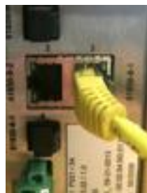
Figure 13 : Ethernet connection plug (M2-J3)
