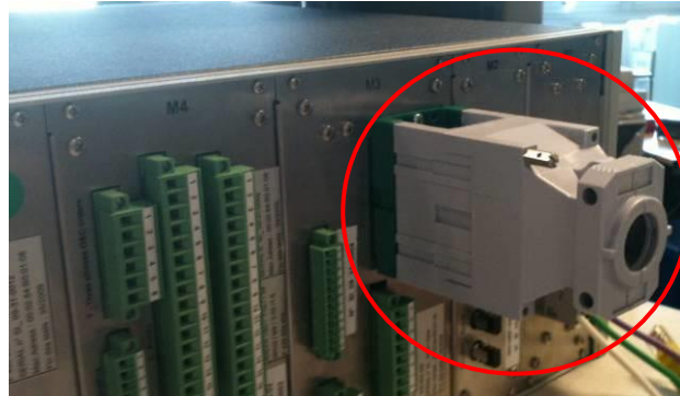
Figure 40 : safety socket on M3-J4 interface
